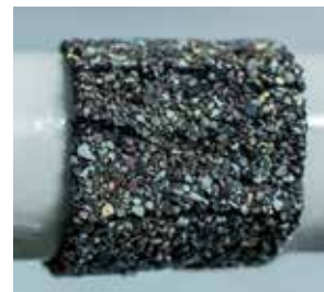
non-modified asphalt shingle with cracking
